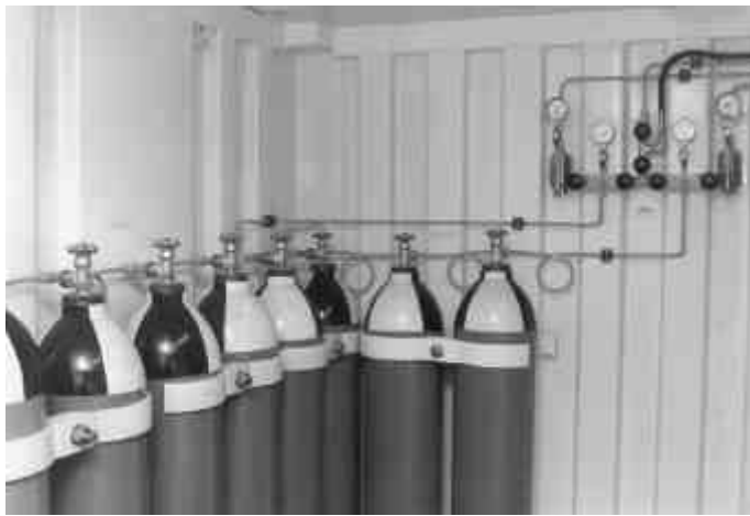
Part of a high pressure air bank, complete with distribution manifolds, with reducers, etc.
