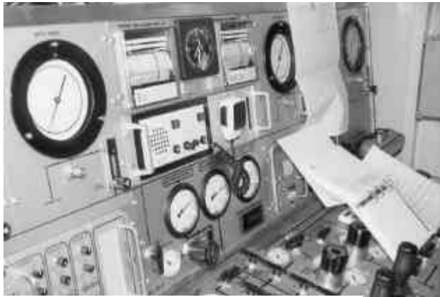
Control and support center for the wet-bell.
